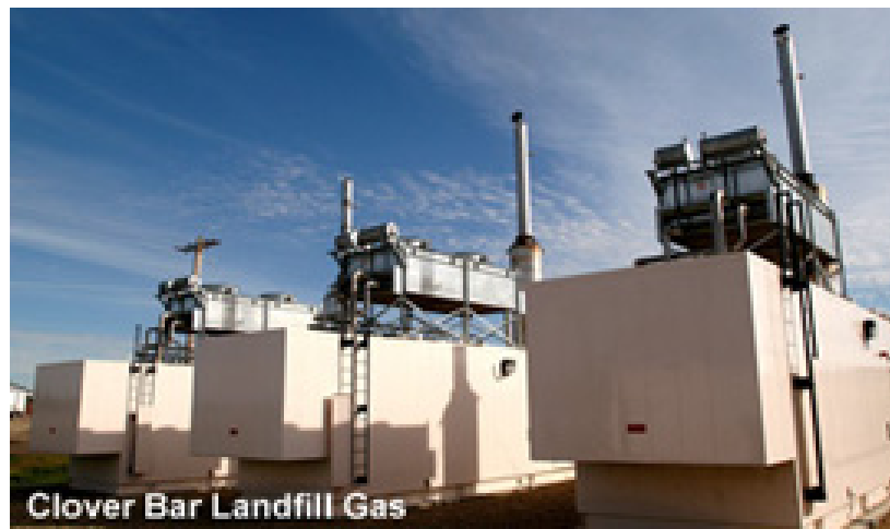
Cloverbar Landfill Gas Facility
