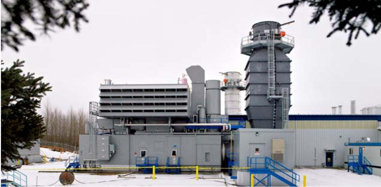
Valleyview Gas Turbine Facility
